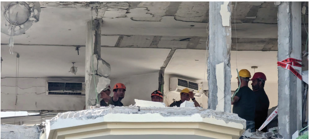
Surveying the damage to Rehovot apartment building following the rocket attack
